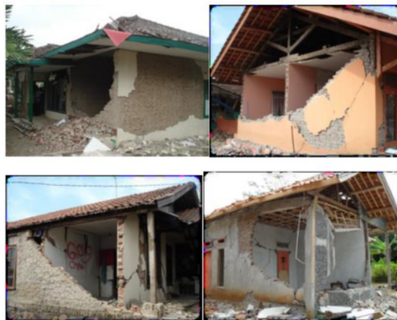
Fig 1: RC frame buildings with burnt clay bricks as infill walls are considerably vulnerable under seismic loadings
